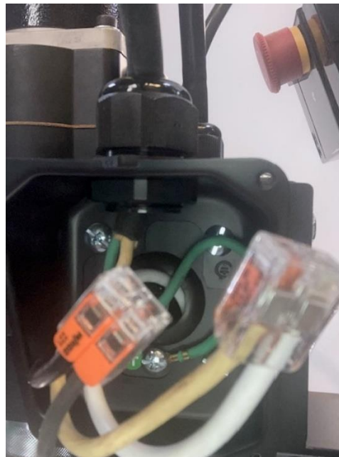
Fig. B. Installed Wiring
